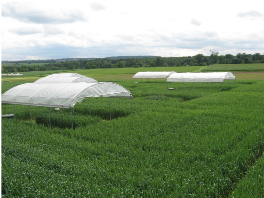
Figure 4: and the view after the installation of the roof (picture from Christian Poll)
